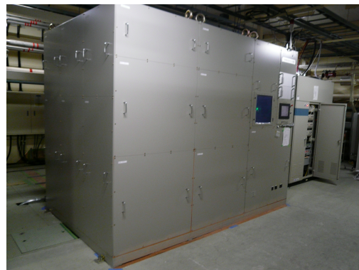
Figure 4: Picture of the power supply at the Linac Klystron gallery
