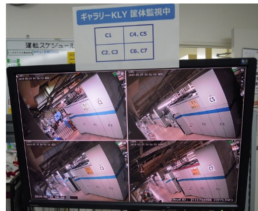
Figure 2: Surveillance video of klystron power supply.
