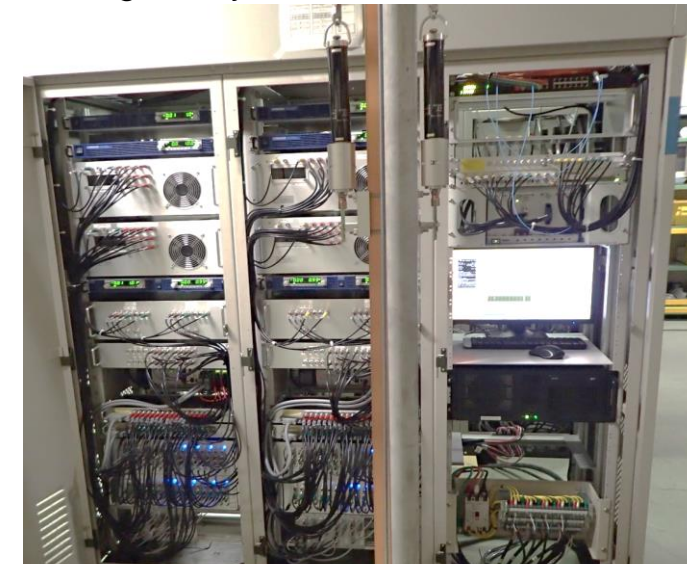
Photo of control unit and power supply
