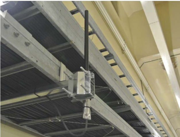
Figure 7: Installed collinear antenna at the KEKB tunnel linear section.
