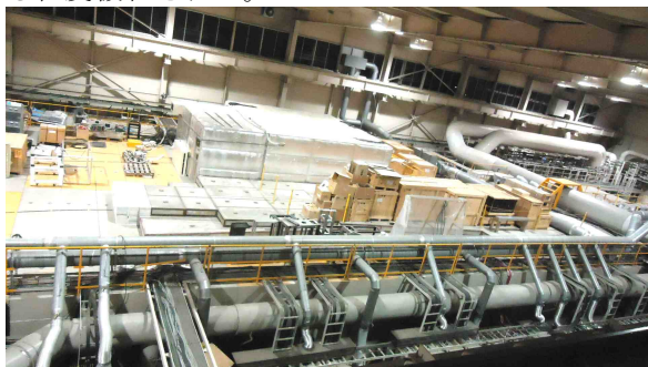
Figure 3: Ventilation ducts for cooling the floor of the DR
