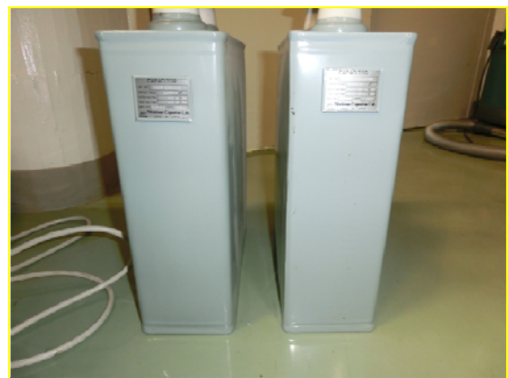
Figure 6: PFN capacitors. Left: damaged, Right: new.
