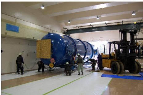
Figure 4: Location movement of the accelerator tank by electric movable carriages.
