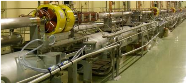
Figure 14: Hydrostatic leveling system.
