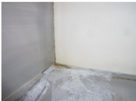
Figure 2b: Closeup of a location of water-leak (D10-B).
