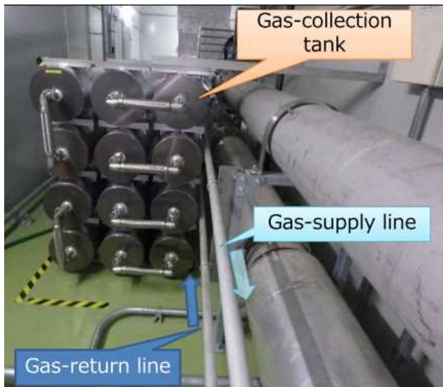
Figure 4: Photographs of the gas pipes and the gas-collection tank in the sub-tunnel.
