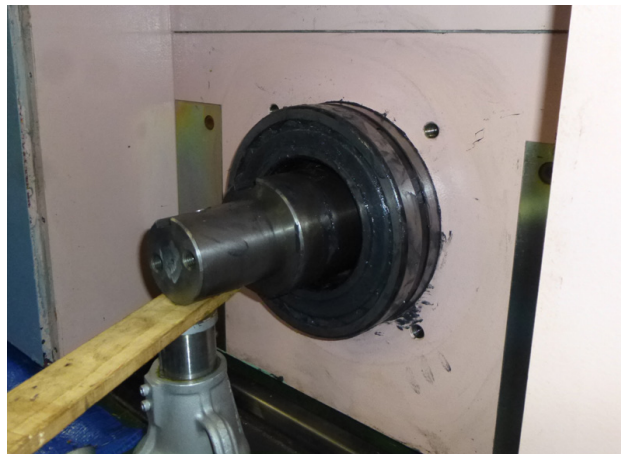
Figure 3: Replacement of a bearing used in a shielding door.
