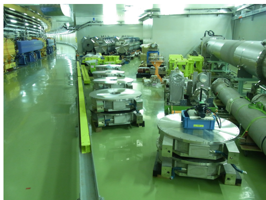
Figure 3: 10 recycle tanks installed FT3M cores.
