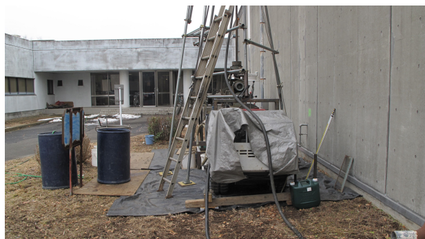
Figure 2: Preparation of boring devices and a boring point in the 17.6 m north from the entrance of the injector linac building.
