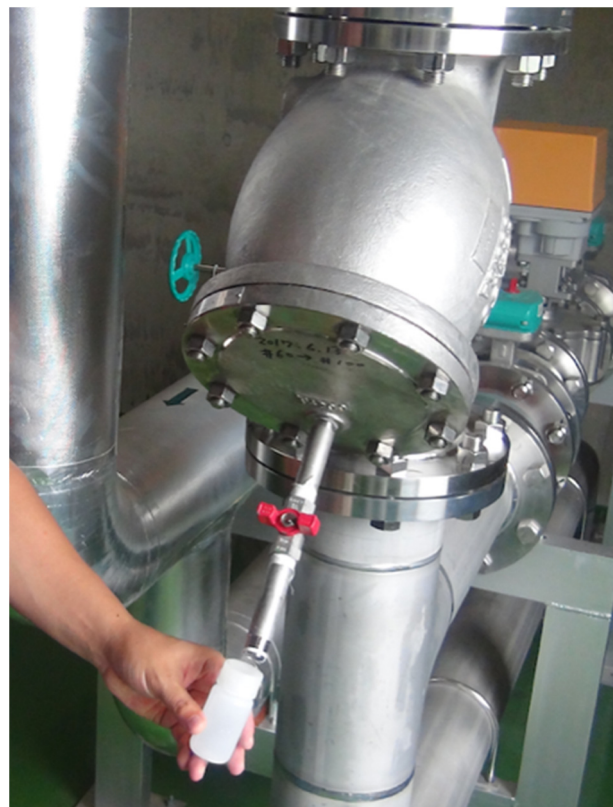
Figure 6: Strainer drain near the three-way valve.
