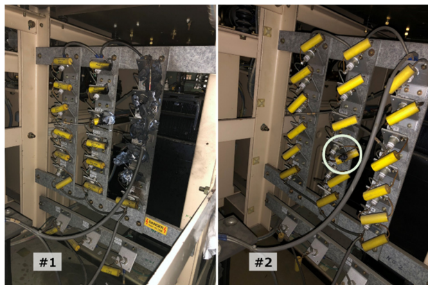
Figure 3: The high voltage regulator units for the high speed voltage stabilizers in the modulator dc power supplies.
