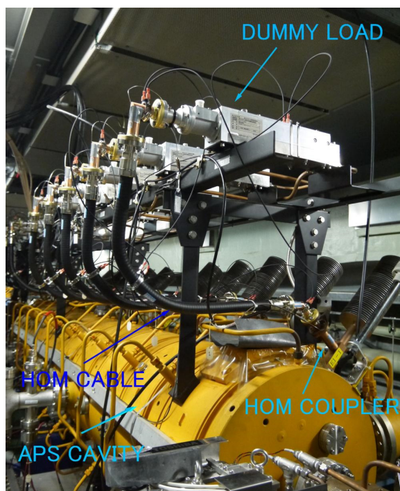
Figure 7: Picture of the renovated HOM cable system.
