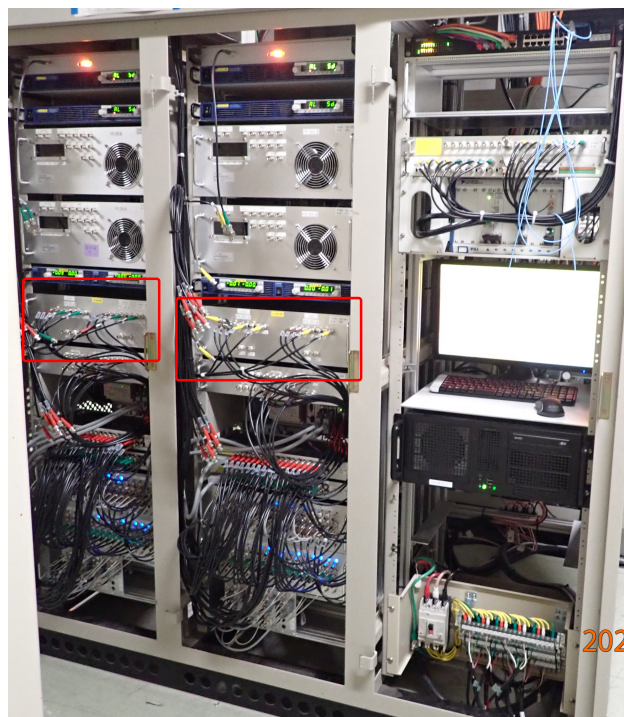
Figure 1: Power supply system for pulsed magnets. In addition to pulsed power supply, control system, interlock system, DC power supplies for charging capacitors of the pulsed power supplies are shown. Each unit feeds 8 ch pulsed magnets. Bipolar power supplies for pulsed steering magnets are indicated by red rectangles.
