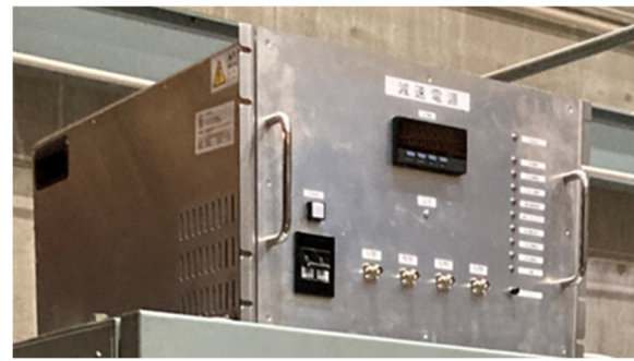
(a) Appearance of New deceleration power supply
